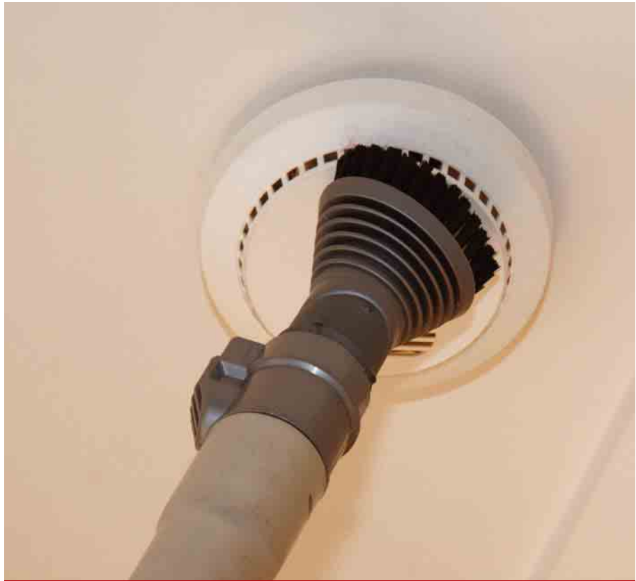
Dust smoke alarm with vacuum cleaner
